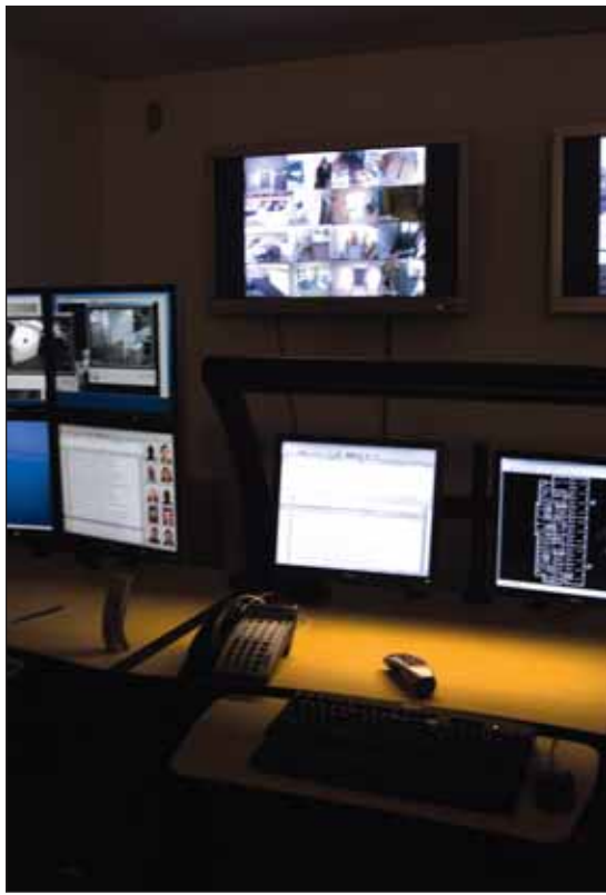
The command and control center features four 20-inch monitors for 100 cameras. Another 200 will be added as construction continues. Alarms generate video displayed on one of two 42-inch plasma screens. All card reader activity is also displayed, along with the associated employee photo.
